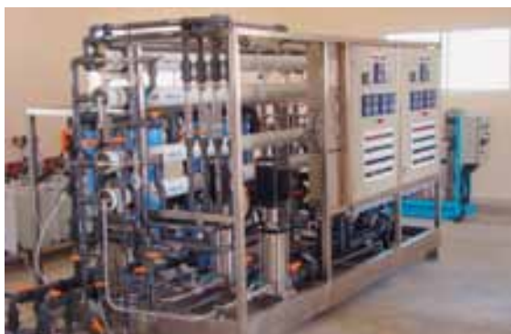
■ Water treatment facilities in Dhahboun
