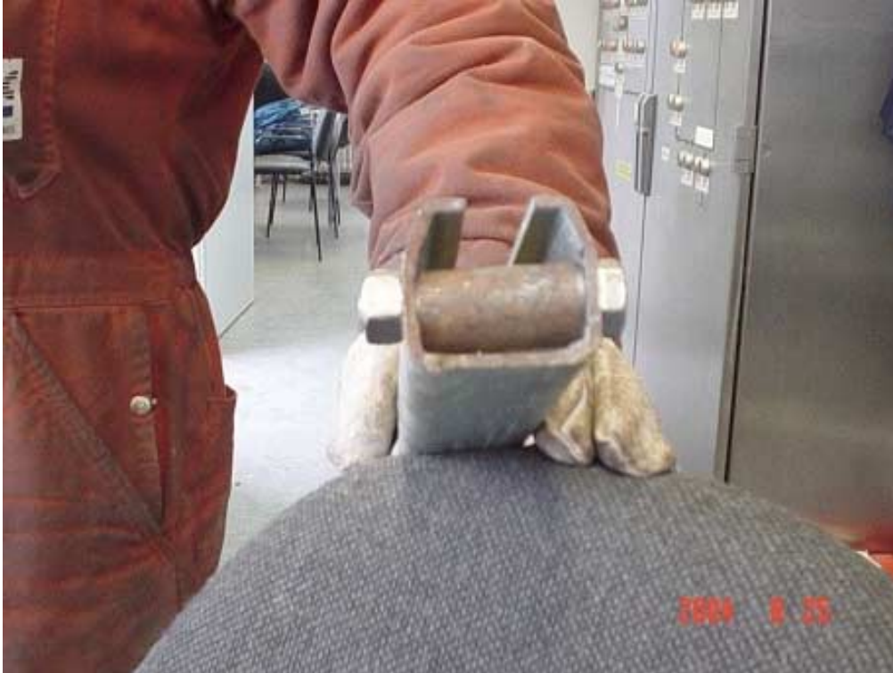
End stopper in the sliding door rail as modified at T-2000
