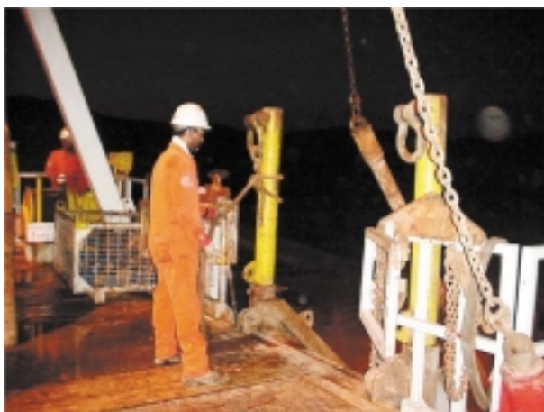
WRONG : In front of DP
