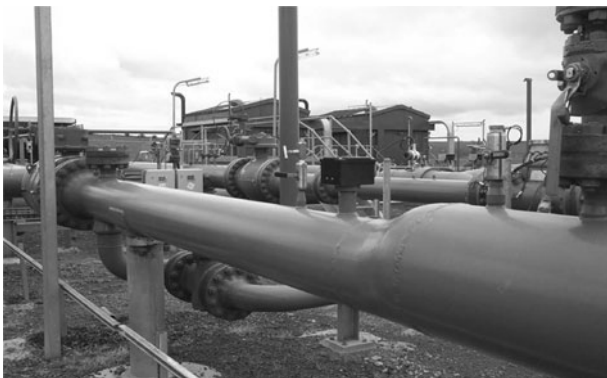
FIGURE 1: SHOWING MAIN ISOLATION VALVE ON LEFT AND THE SECOND PIG SIGNAL DEVICE (BLACK BOX ON TOP OF RECEIVER BEFORE TRANSITION SECTION)
