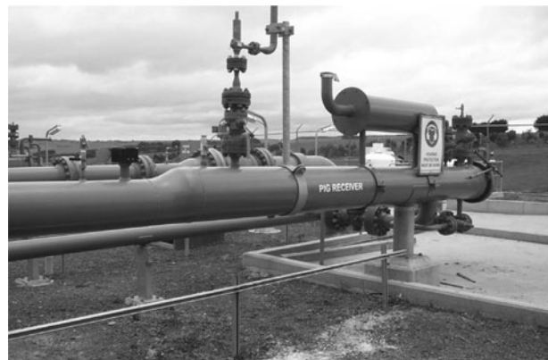
FIGURE 2: SHOWING, FROM LEFT TO RIGHT, SECOND PIG SIGNAL RECEIVER, TRANSITION SECTION, PSV, VENT AND VENT VALVE, AND RECEIVER DOOR
