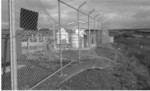
FIGURE 3: SHOWING DAMAGE TO THE PERIMETER FENCE
