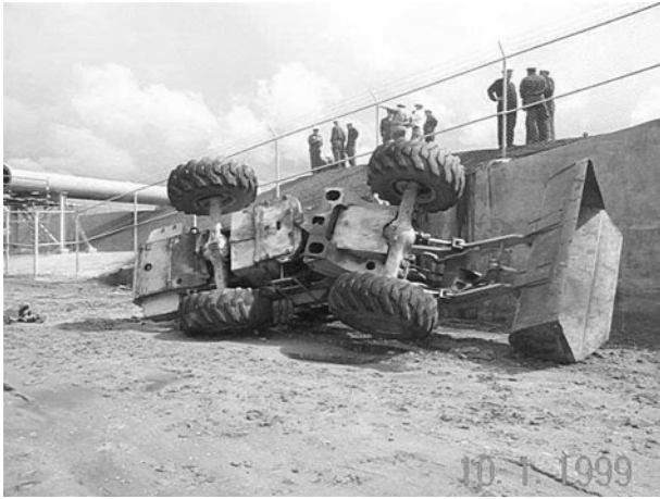
FIGURE 5: THE LOADER AFTER FAILING TO CATCH THE PIG
