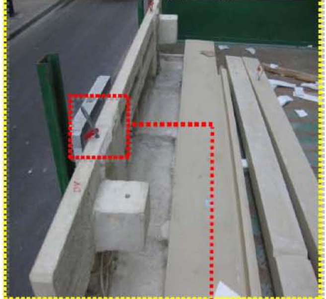
GRC panel is to be lifted by tower crane attached to two (2) lifting points
