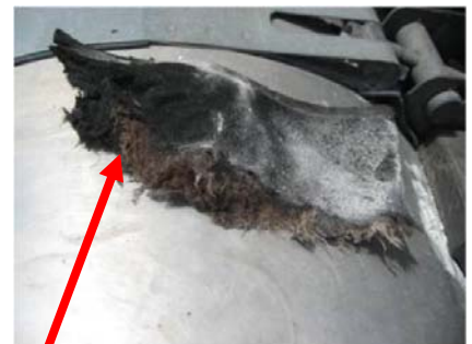
Remains of damaged insulation
